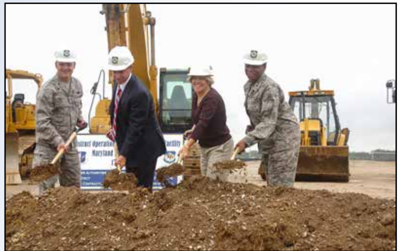
Brig. Gen. Allyson Solomon and Brig. Gen. Scott Kelly, along with two civilian representatives, toss a scoop of dirt, officially kicking off the construction of the new wing headquarters, operations, medical and training facility.
