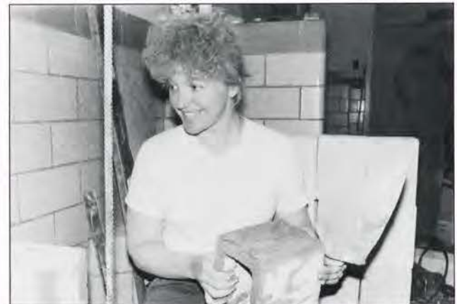
BUILDING BLOCKS: Staff Sgt. Anita Hart, a 120th Civil Engineering Squadron, Montana Air National Guard carpentry specialist, does double duty as she prepares to set a cinder block on a shower room wall during dormitory remodeling at the Montrose Military Reservation. (Photo by Capt. Mike Milord)
