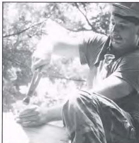
HIGH CONSTRUCTION: Completing the frame on one of 20 Adironek shelters at Montrose is a 121st Engineer Battalion construction specialist. (Photo by Capt. Mike Milord)
