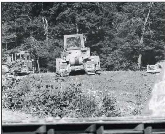
Members of the 243rd Engineer Company assist in the construction of a ballfield at Beall High School in Frostburg, Maryland in June 2001.
