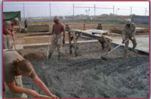
Soldiers with the 253rd Engineer Detachment work on a foundation while serving in Afghanistan in support of Operation Enduring Freedom.
