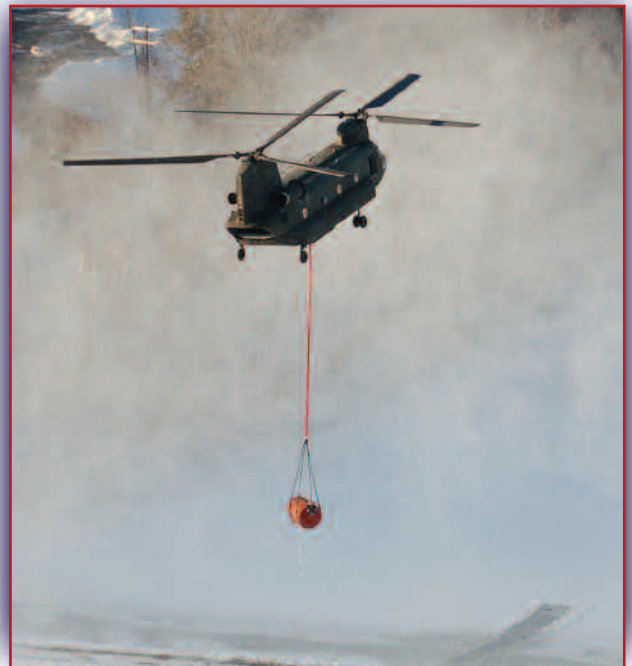
A Maryland Army National Guard CH-47 Chinook helicopter is used to hoist a diesel fuel tank into position on top of the Oakland Dam.
