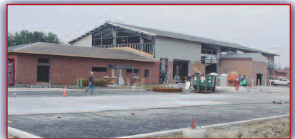
The Dundalk Field Maintenance Shop at 60% completion. When operational, by the summer of 2008, the shop will support Maryland Army National Guard units throughout the Baltimore area, increasing readiness for state and federal missions.
