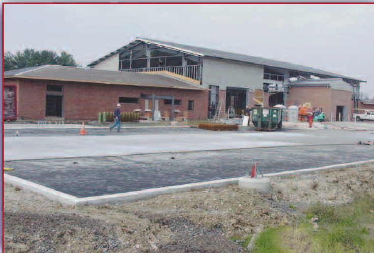
The Dundalk Field Maintenance Shop is at 60% completion. The shop will be operational by the summer of 2008.
