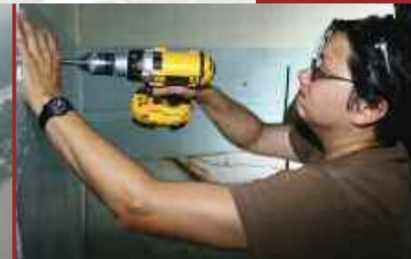
Master Sgt. Cathy Burns, a member of the Maryland Air National Guard's 175th Civil Engineer Squadron, drills a hole for mounting a light switch at a primary school in Vlasenica, Republika Srpska, Bosnia-Herzegovina July 15, 2008, as part of a humanitarian civic action project under the auspices of the National Guard's State Partnership Program. (U.S. Air Force photo by Capt. Wayde R. Minami)
