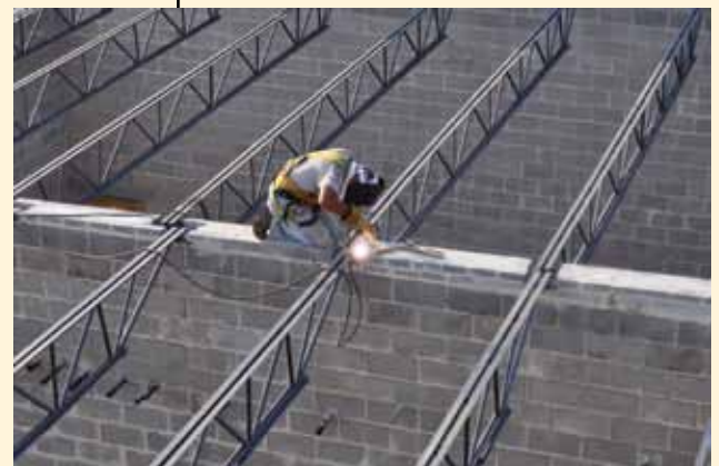
A construction worker works on the structure of the new addition to the Salisbury armory. The addition to the armory utilizes various types of environmentally friendly techniques such as the utilization of innovative wastewater technologies.
