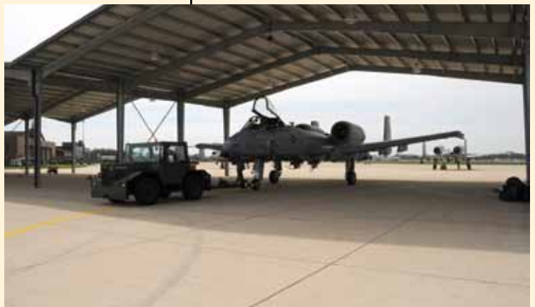
New sunshades installed at the Maryland Air National Guard, 175th Wing at Warfield Air National Guard Base in Baltimore, Md., April 21, 2011. The sunshades are design to help keep maintenance costs down. The shades will also protect the aircraft from rain, hail, snow and UV rays that can deteriorate gaskets, rubber seals, paint and other items costing more to maintain aircraft.
