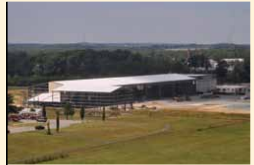
The Maryland National Guard's Army Aviation Support Facility receives a new addition to the flight facility, as well as a renovation to the existing facility on the Edgewood Area of Aberdeen Proving Ground, Md. The addition will bring space for an administrative area, equipment storage areas, classrooms, a physical fitness area and modernized shops to support Army aviation and maintenance.
