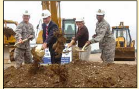
The Maryland Air National Guard kicked off the construction of the new facility that will consolidate the location of the 175th Wing Headquarters personnel, Mission Support Group and the Medical Group, Oct. 2, at the Warfield Air National Guard Base in Middle River, Md.
