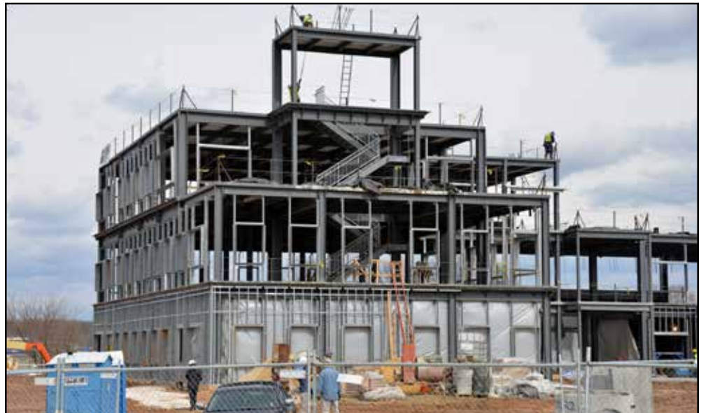
The last installed I-beam completes the shell of the new 175th Wing Headquarters, Mission Support Group and Medical Group facility at Warfield Air National Guard Base, Middle River, Md. February 28, 2013. This new construction has a projected cost $11.8 million, and features multiple green roofs and is anticipated to achieve certified LEED Silver status with the numerous energy enhancement measures upon its completion. Functional areas include offices, medical/dental examination and treatment space, classrooms, administration space, command section, conference rooms, telephone switching/data automation center as well as utility systems services and connections.
