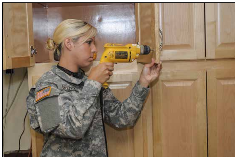
A 60-year-old fire station in Mount Washington had its kitchen renovated free-of-charge, minus the cost of supplies, by a dozen members of the 244th Engineer Company from the Maryland National Guard looking for rehabbing experience prior to an Afghanistan deployment.
