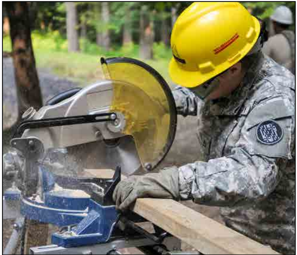
Soldiers from 2nd platoon, 244th Engineer Company, Maryland Army National Guard, broke out the hammers and circular saws to repair the Leadership Reaction Course at Gunpowder Military Reservation in Glen Arm, Md., August 3-11, 2014.
