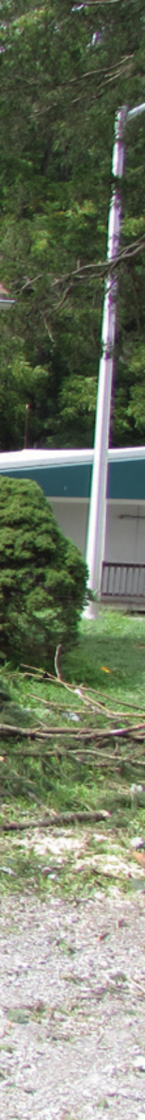
MDDF Engineers conducted tree removal operations at the Camp Fretterd Military Reservation saving thousands of dollars.
