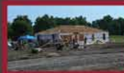
Airmen of the 175th Wing, helped finish construction on homes built for Cherokee Veterans.
